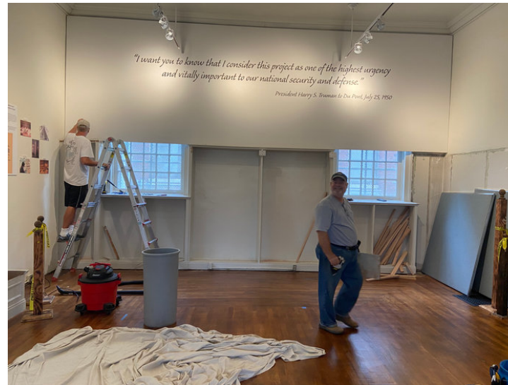
(Image 4) Andy Albenesius, Chairman of the SRS Heritage Foundation (left), works to remove a section of bookshelf on the North Wall. David Wilkerson (right) removes debris.
