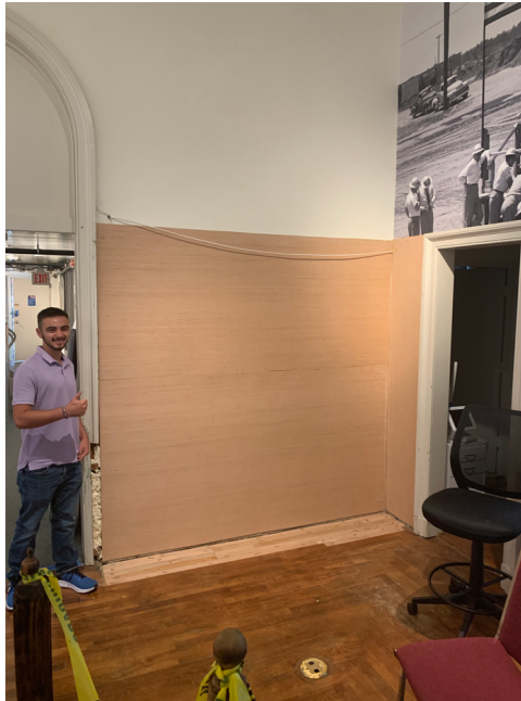
(Image 5) Ches Mathis, SRS Museum intern, poses beside a newly paneled wall.
